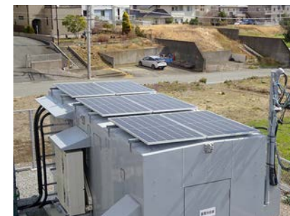
Container-type green base station (Shizuoka Prefecture)
