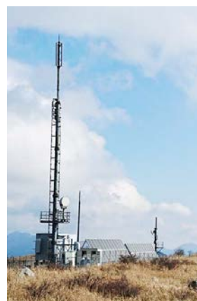
Fuel cell installed at the Nomura Ohnogahara Green Base Station in Ehime Prefecture
