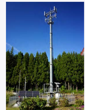
Green base station
