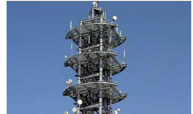
Large-zone base station that secures communications in densely populated areas in times of disaster
