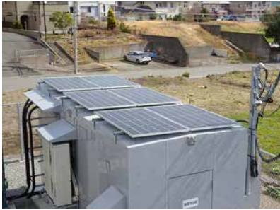
Container-type green base station (Shizuoka Prefecture)
