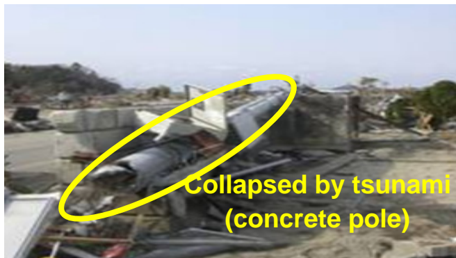
(1) Base station facility (Matsushima-Nobiru, Miyagi Pref.)
