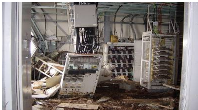
(3) Transmission equipment (Noda, Iwate Pref.)
