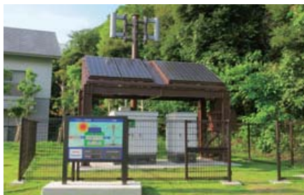
Green base station
