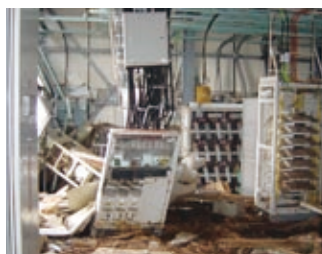
Telecommunications equipment (Noda Mura station in Iwate Pref.)
