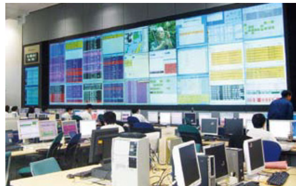
At the DOCOMO Network Operations Center, base stations and circuits are monitored and controlled 24 hours a day, 365 days a year.
