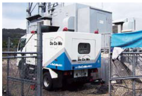
Restoration of base stations through mobile power generation vehicles
