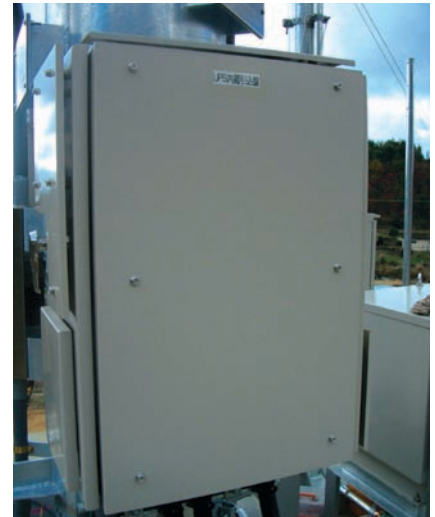
Photo 1 External view of outdoor booster equipment
