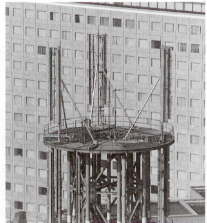
図3 3セクタ用ダイバーシチ受信構成アンテナ配置 Figure 3 Installations of Diversity Reception Antennas for Three-sector Zone Use
